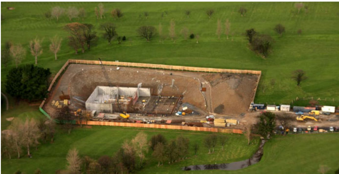
Figure 2-8: Irish Water Underground Foul Water Storage Tank
